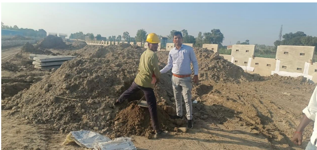
Figure 1. Site of the field trial RE wall construction. Precast concrete facing panels (with connection slots) are positioned, and the local soil is sampled for characterization prior to stabilization.
