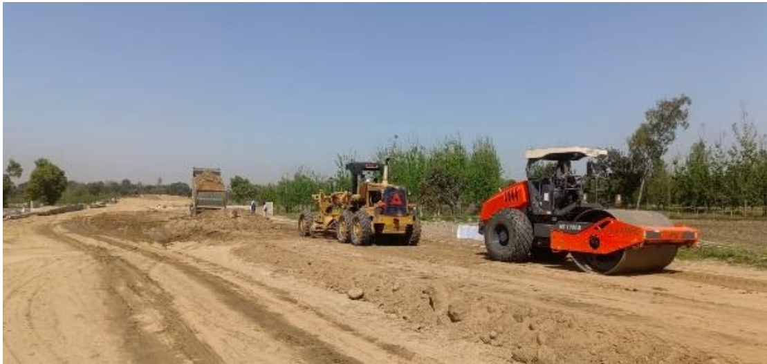
Figure 2. Field compaction of the slag-fiber stabilized backfill using a vibratory roller. Fewer compaction passes were required compared to conventional soil due to the improved compaction characteristics of the mix.
